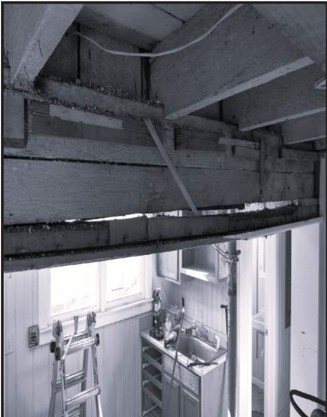
Deteriorated kitchen beam carrying 2nd floor.
